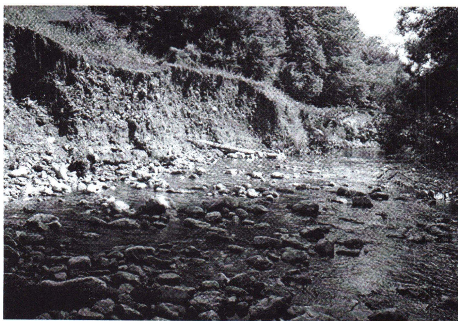
Fig. 1 Miodrag Babic (Babica Mala hamlet) pointing out the damages caused by the rising of water current, which has, moving its riverbed, almost halved a part of the parcel by the riverbed
